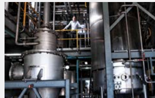
2007 MACKAY PILOT PLANT
